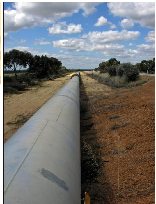
The Kalgoorlie pipeline is the longest freshwater in the Southern Hemisphere!
